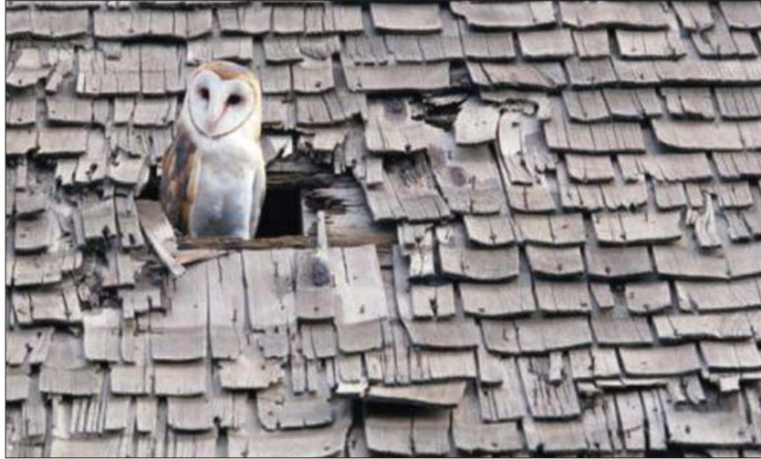
Example of Property Standards Violations
